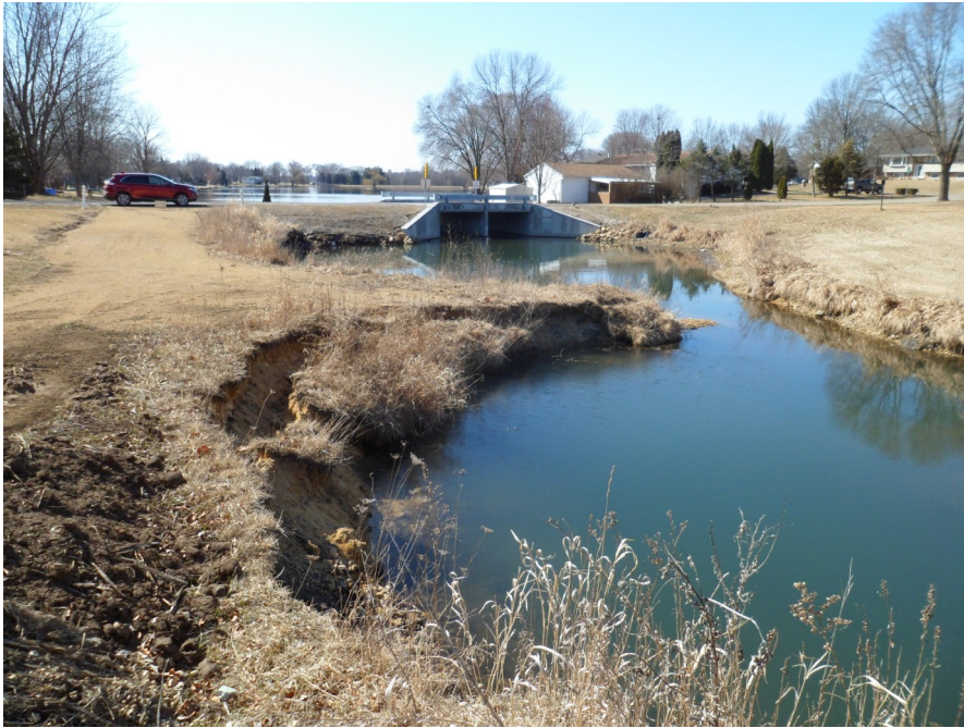
North Catchment, Pond East wall ~ Partial collapse.
