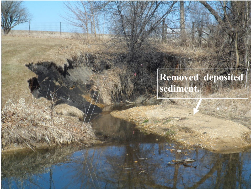
Before repair. Feeder stream, partial collapse of west bank. The stream had changed course and deposited sediment. When the stream level was high the sediment deflected the water flow against the west bank causing the collapse.
