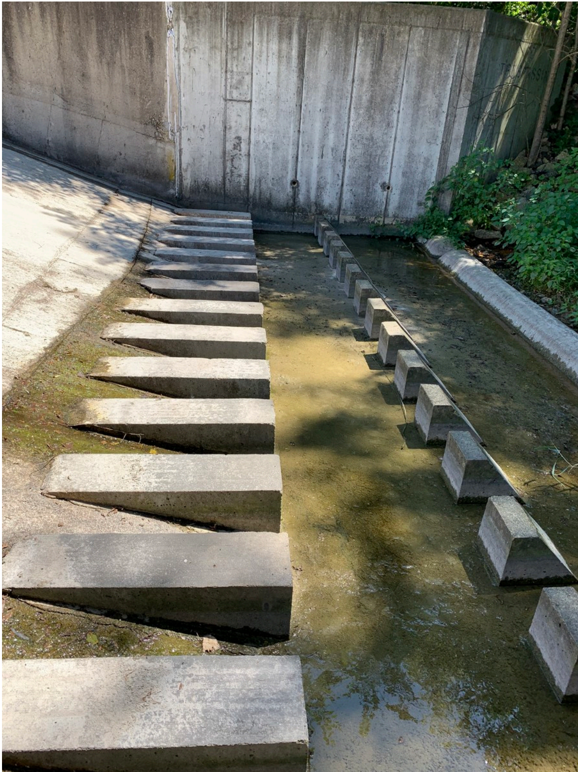
Photo #5 – Emergency spillway energy dissipator. Minor seepage from spring at slab joint.
