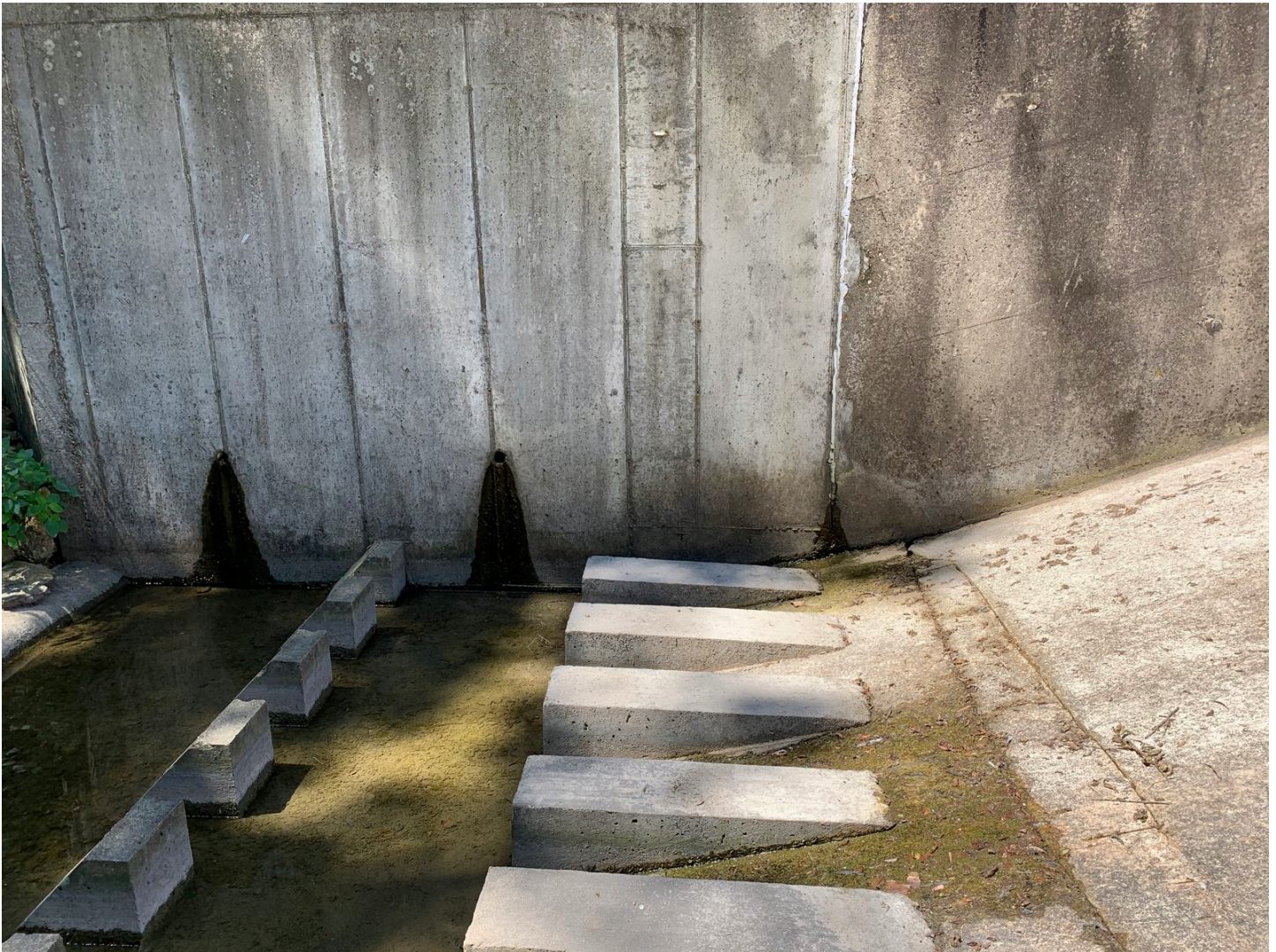
Photo #6 – Minor seepage from spring at bottom of wall joint and active weep holes.
